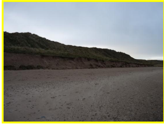
E52/5 – Substantial and consistent toe erosion, but little evidence of instability in the upper cliff. This level of erosion was consistent throughout the unit. December 2013 (Locally Active).
