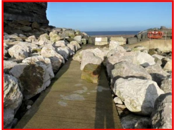
MU4/1a - Displaced rock armour and rockfall block on path after the December 2013 surge. (Totally Active)
