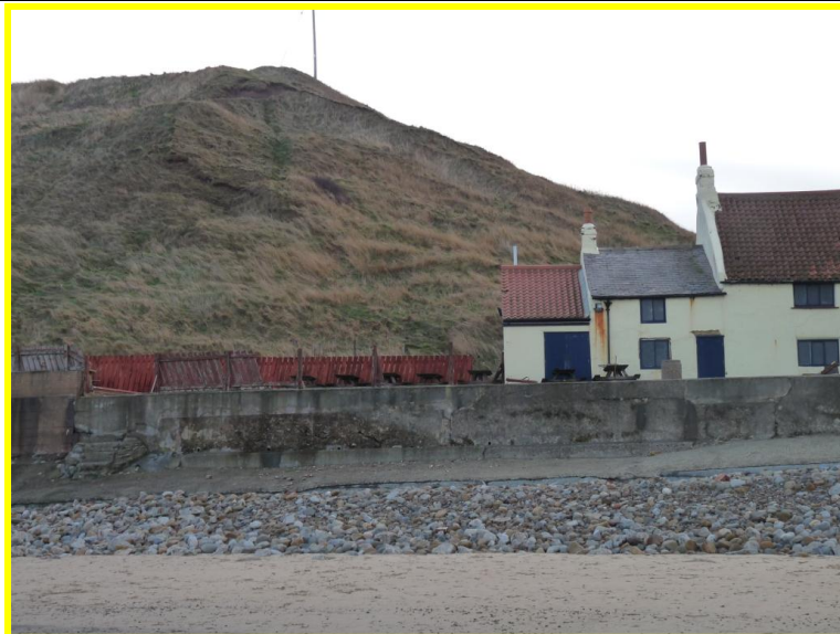
E53/5 – Slump identified in previous survey not yet completely revegetated therefore ‘Locally Active’ Status has been retained. December 2013
