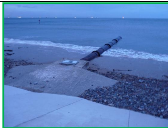
MU52/11 – Exposed pipe (one of several). Provides reference for beach level.(Dormant)
