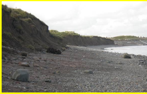
E52/10 Interface between new seawall and cliff at Mill Howle (Locally Active) October 2012
