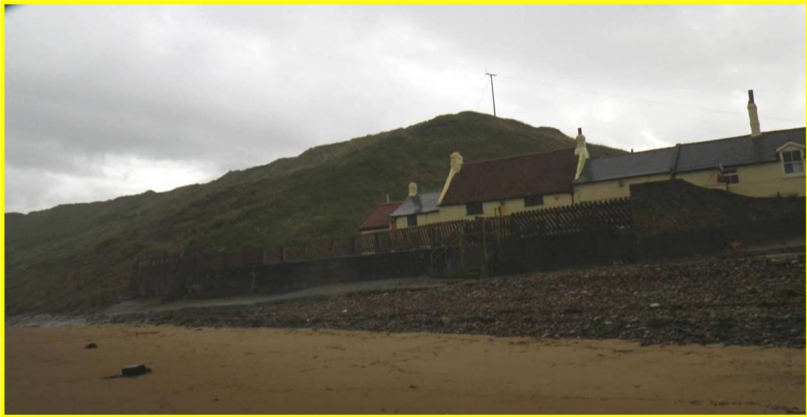
E53/5 has slumped, leaving open cracks in the cliff face and resulting in instability classified as Locally Active. September 2012
