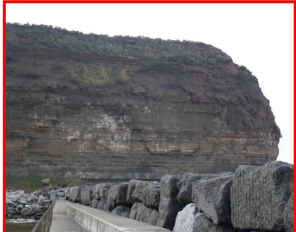
E60/1a - The northern half of Cowbar Nab. The cliff face is showing signs of erosion (Totally Active) Sept 2012
