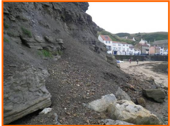
MU4/2 – There have been a number of recent failures in this management unit, which is now classed as Partly Active. Sept 2012
