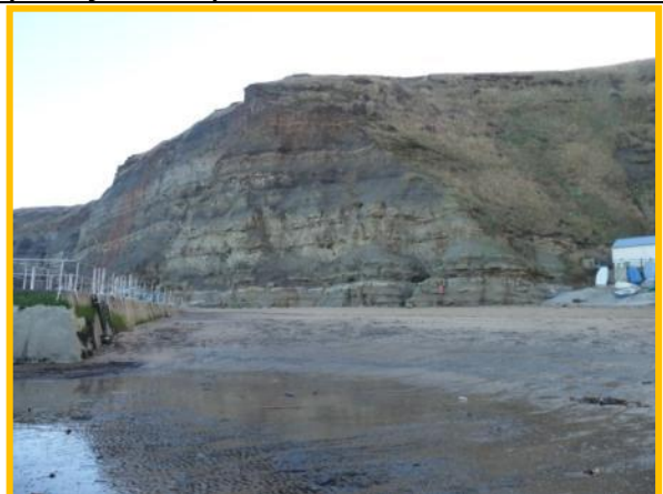
MU4/2 - Beach condition post December 2013 storm surge. Note absence of talus at base of cliff. (Partly Active)
