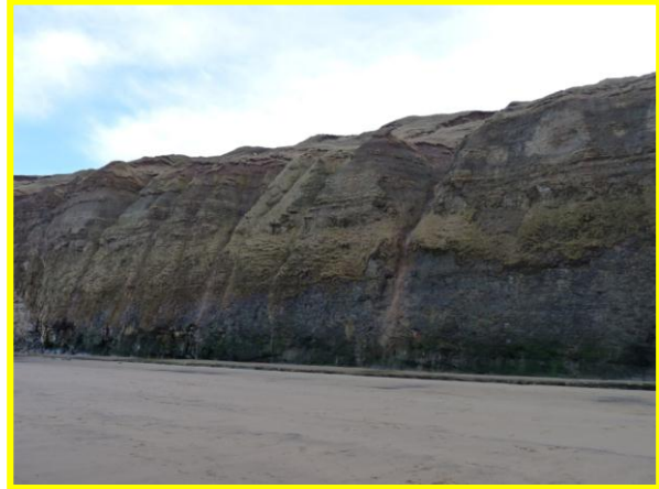
E53/3 – Central part of unit. December 2013. Note streaking down cliff due to erosion/failure of till. (Locally Active).
