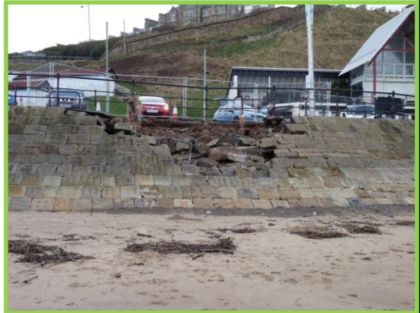
E52/2 – Sea wall damaged during storm surge at toe of E52/2. December 2013. (Inactive)
