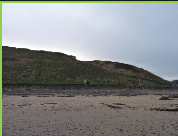
E52/3b – Stabilised slopes with no evidence of instability. However, damage to sea wall experienced during surge as indicated by ongoing repairs. December 2013. (Inactive)
