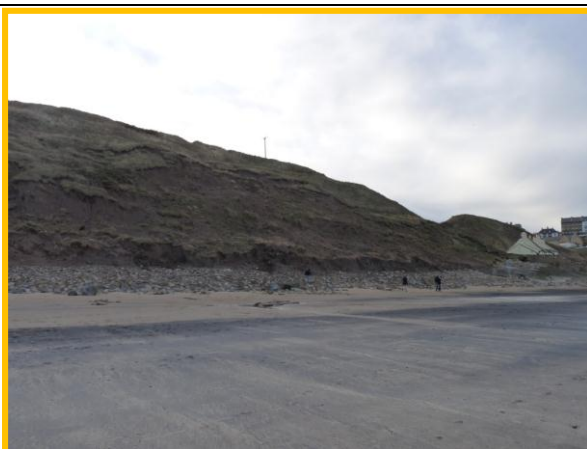
E53/4 – Continued slumping of the till cliffs (northern end of the unit). Toe erosion has been consistent throughout the unit and therefore the activity status has been elevated to Partly Active. December 2013.
